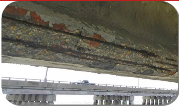
Poor (Structurally Deficient)
